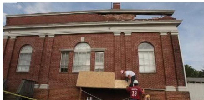
Workers begin repairs Wednesday on the Mineral, Va., City Hall after it was damaged by Tuesday's 5.8 earthquake.
