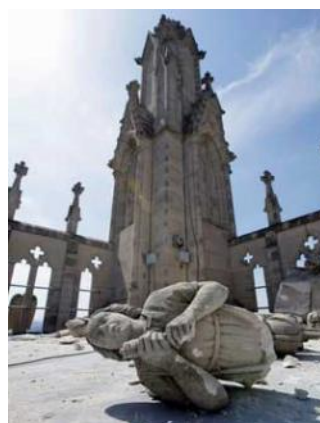
An angel, carved from Indiana limestone, lies shattered on the roof of the National Cathedral in Washington after Tuesday's earthquake.
