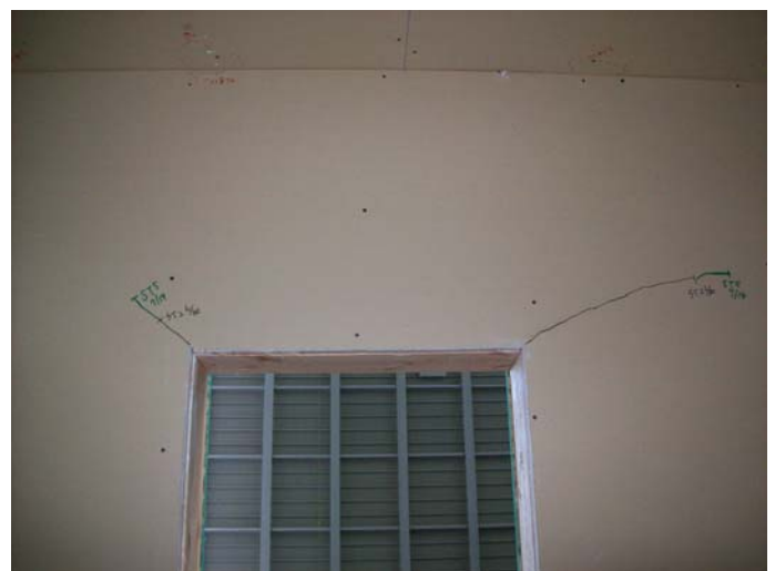
45 degree cracks at corners of window opening
