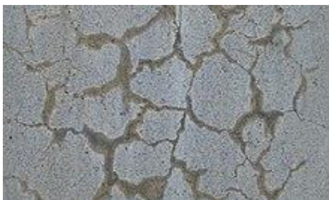
Cracking due to ASR (Wikipedia)
