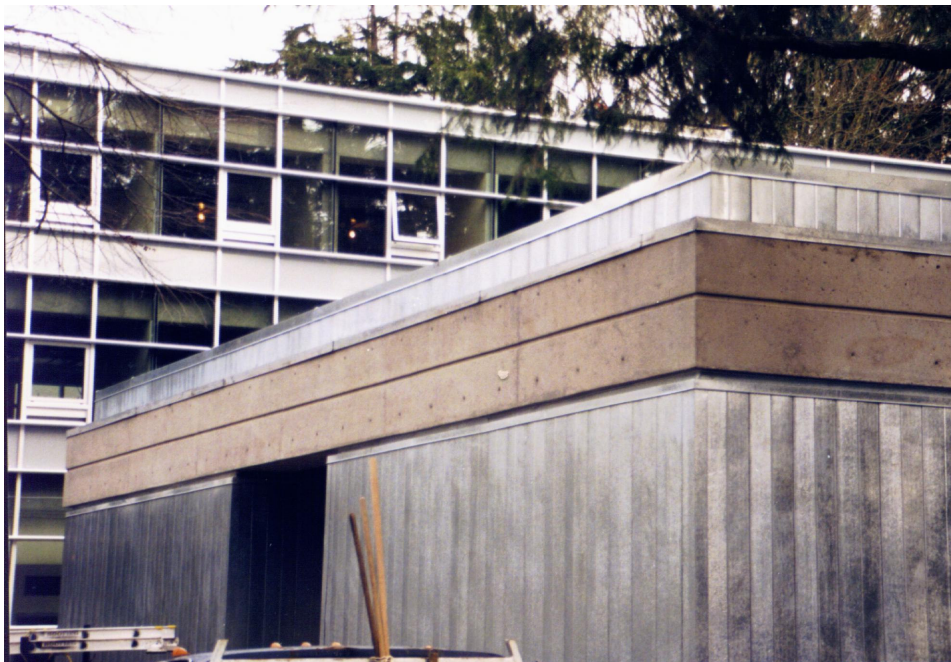
Photograph 2 The HVFA Concrete used in the Liu Centre produced a high quality concrete with a slight “pinkish” tone.
